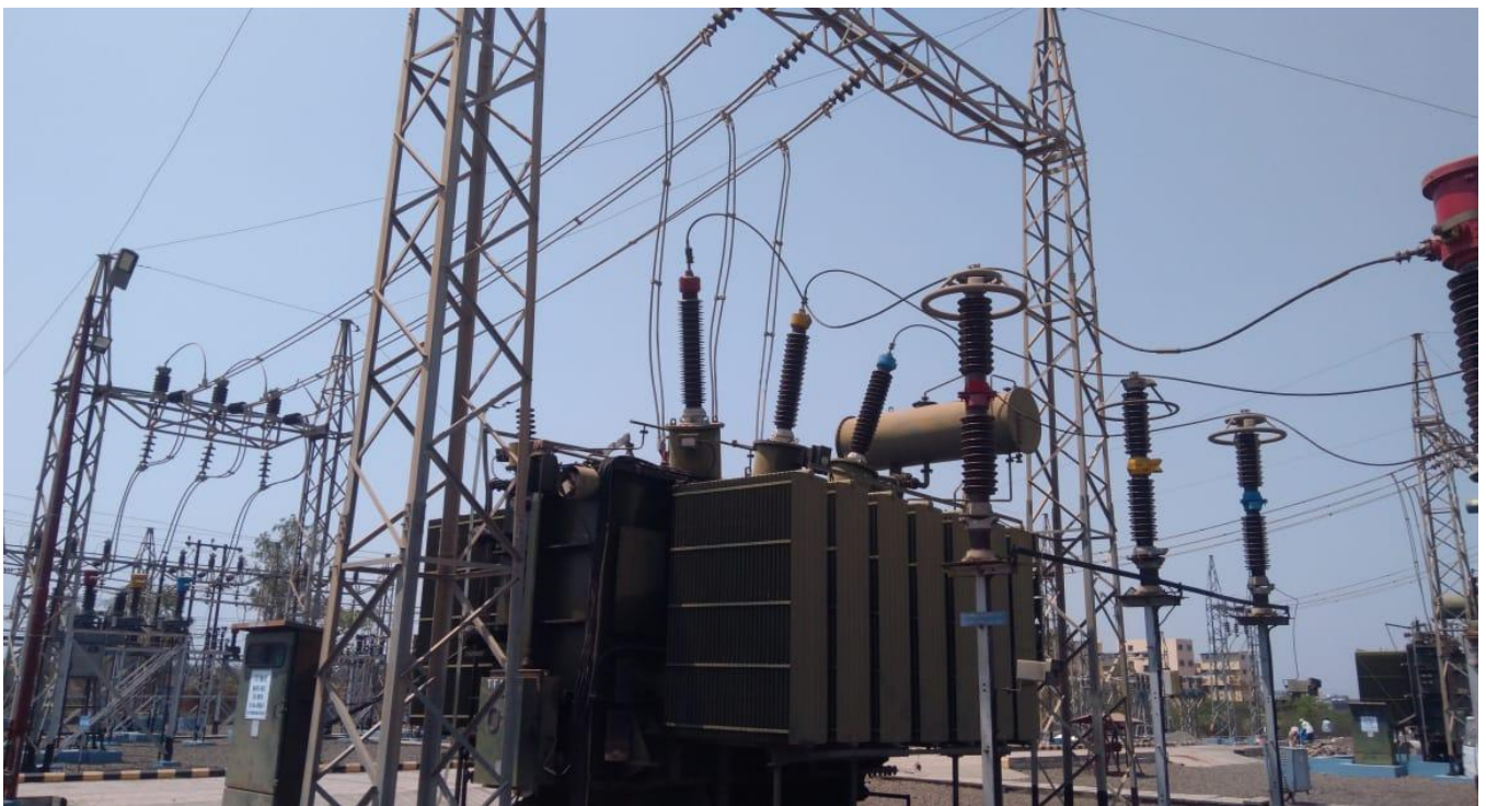
Transformer 110kv/ 33kv in the switch yard.
